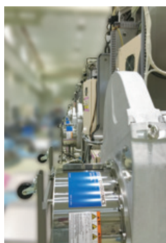
Crypumps installed on Manufacturing Equipment
